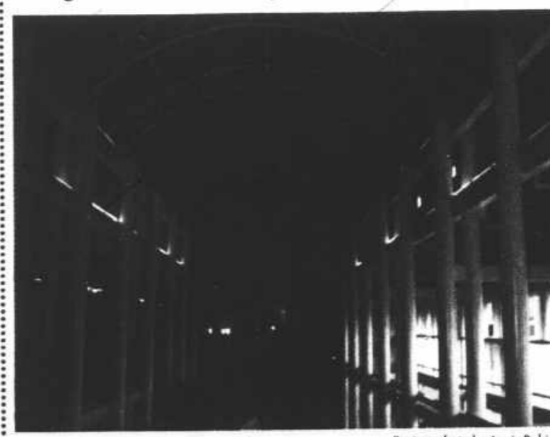
The barrel-vault roof design at the student center may be pleasing, but it hasn't been able to stop occasional leaks.
